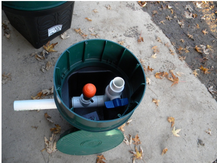
Figure 8. Turn-up and \frac{3}{4} inch air gap/ bleeder at the end of each lateral for routine maintenance
