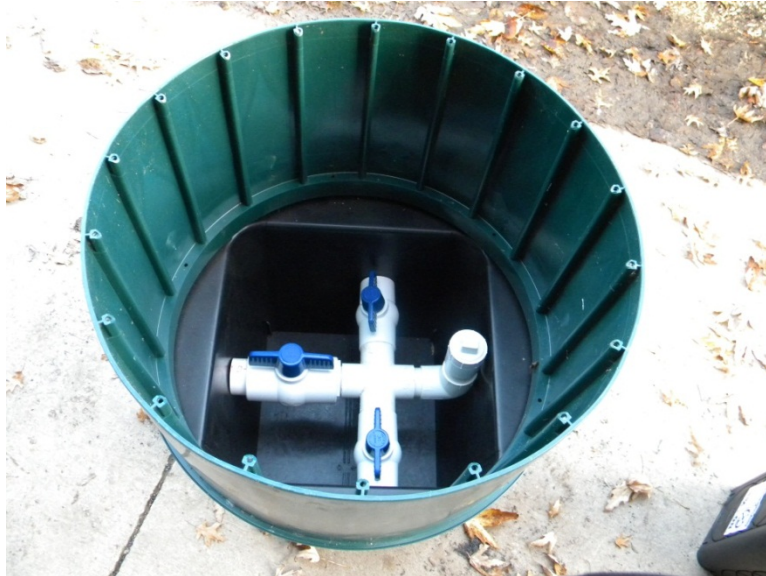
Figure 7. Service box within the manifold line
